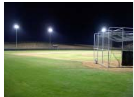
With homes slated to go in soon, the decision was made to move the field lighting to phase one, and baseball was able to play several games under the lights.
